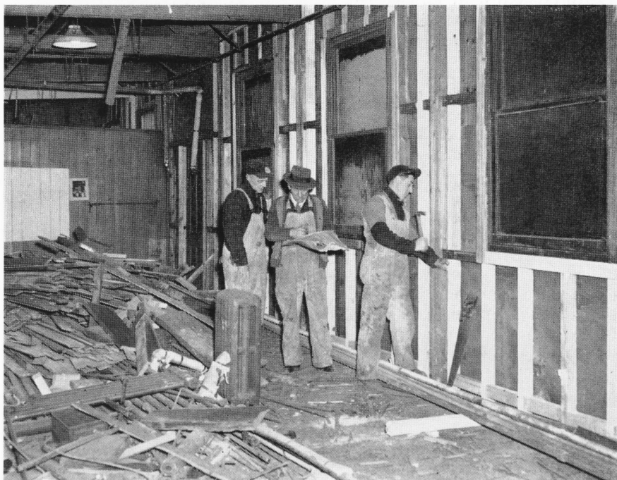
Sixty-one building, along with the Spencer Block at East Main and Mill Streets, is being remodeled to house the entire staff and divisions of the Department of Employee Relations. Here N. C. Stewart, superintendent, with Anthony D'Angelo and Herman Passeck, tear into a wall.
